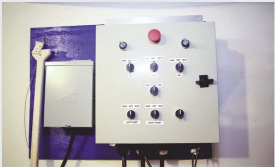
The "brains" of the electric homebrewery come from a unit called a BCS-460, which is produced by a company called Embedded Control Concepts. The unit is controlled via a multitude of processes, switches, relays, and temperature probes incorporated in the system.
