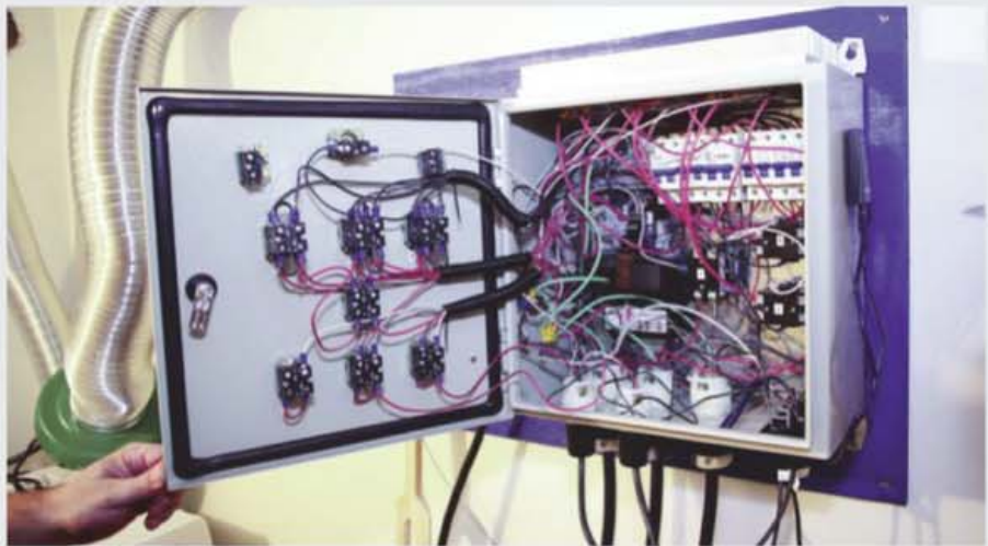
Trent's control panel is a steel NEMA enclosure that is approximately 16 inches wide, 16 inches tall and 8 inches deep (40 cm x 40 cm x 20 cm). This houses the BCS-460 as well as all of the other necessary components needed to control the brew system.
