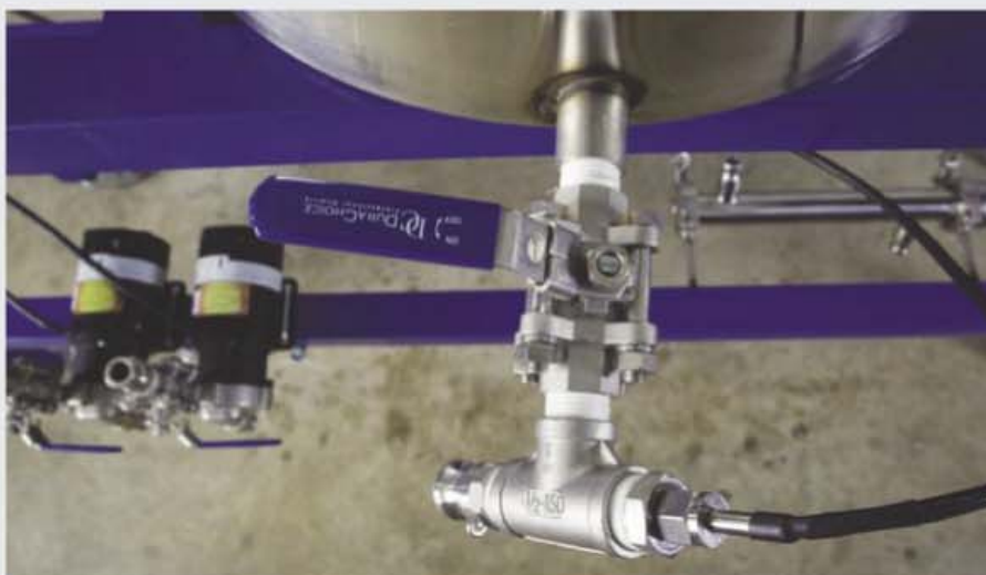
Trent chose to utilize stainless steel three-piece ball valves for his setup, which are easy to disassemble and clean. The advantage to choosing three-piece ball valves over one-piece ball valves is that you run less of a risk of installing the handles out of place.
